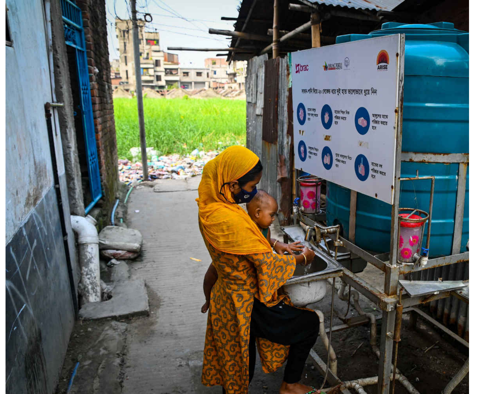
Handwashing devices installed for the community members in Shyampur, Dhaka
